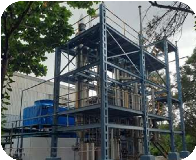
Multiple-effect evaporator and Agitated thin film drier plant
