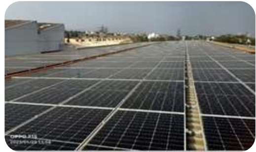
0.41 MW at Padi unit
